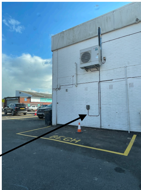
Pic:Example of EV charger installed directly on the wall (qualified for standard installation )
